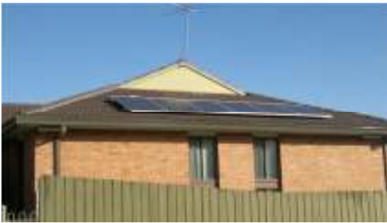
The photo-voltaic (PV) system
